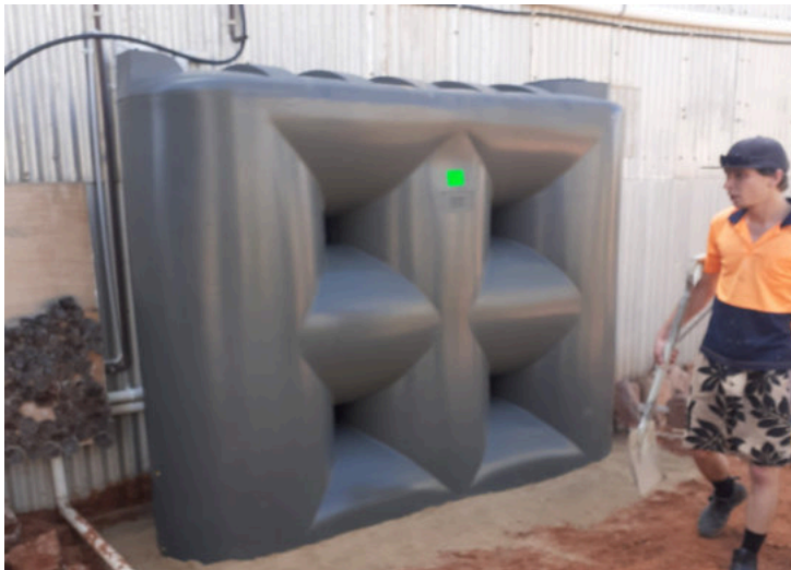
"New splash-pad water tank."
