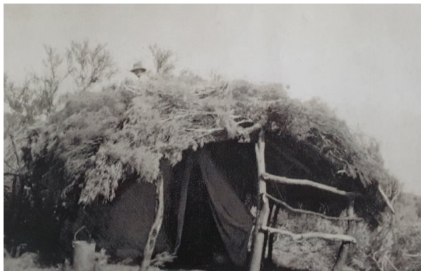
Minnie's Bough Hut is currently being reconstructed with the assistance of the CDP.
