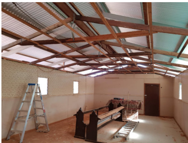
Work has started stripping out the old ceiling and framework to replace with a new insulated ceiling structure.
